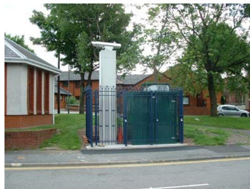
Photo 9 - St Thomas DOAS Receiver Station
