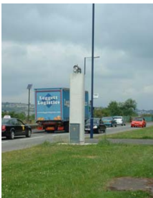
Photo 8 - St Thomas DOAS Transmitter
