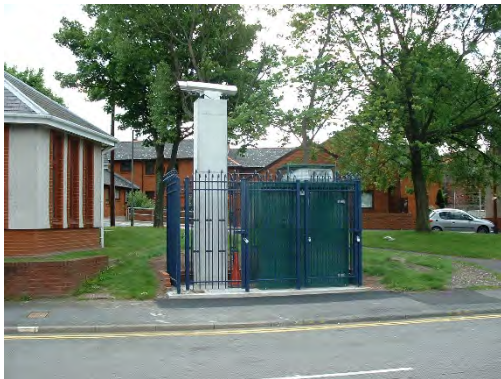
Figure 2.1.1.6 - St Thomas DOAS Receiver Station
